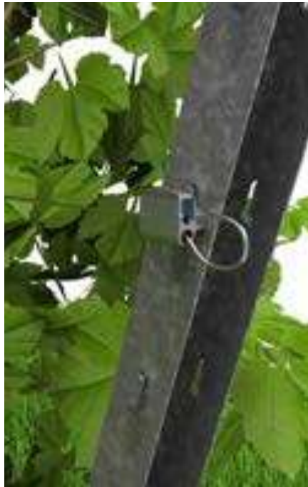
VIT-S - Installed on metal post
